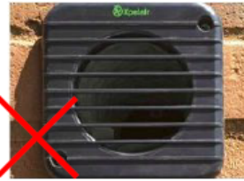
Surface mounted services
