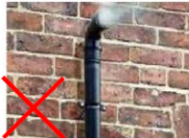
Surface mounted services
