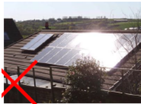
Poorly positioned solar panels
